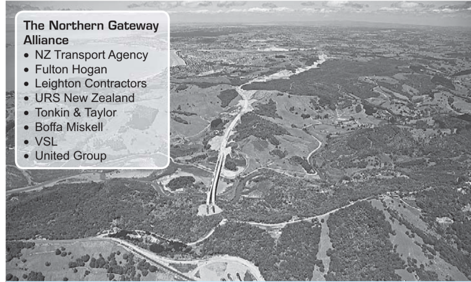
No longer an extension. No longer a hope. Now a reality. The Northern Motorway looking south from Puhoi to Orewa. Photo: Northern Gateway Alliance.
